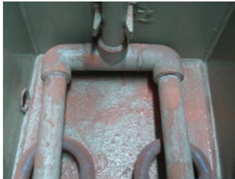
Tank plateout 槽液析出
